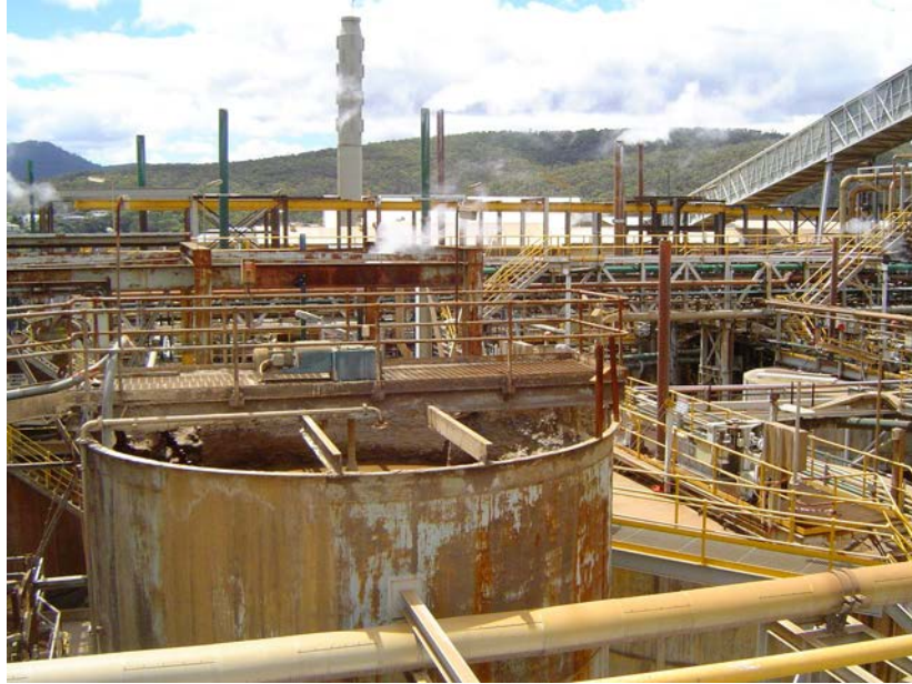
Figure 9 – Reaction tanks and piping in the Leach/Purification Plant
